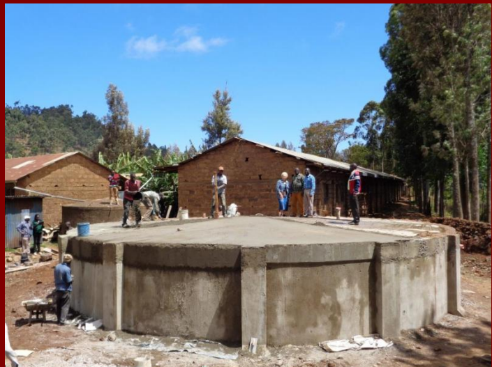
The finished tank at Leeta Primary School. Vickie, Charles, the project contractor, and the school chairman standing on top with the workers.
